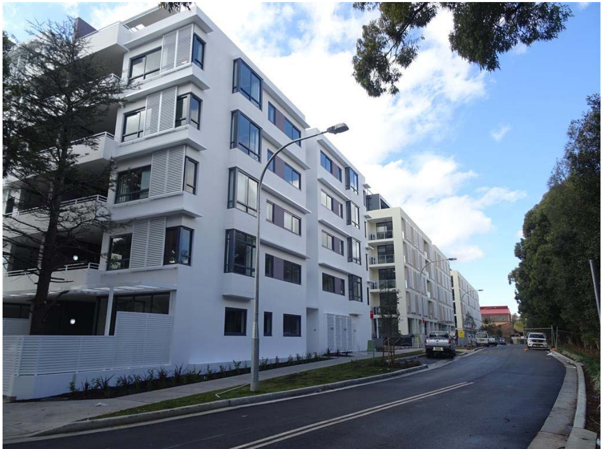
Figure 7: The southern edge of the site showing Buildings D, G and H nearing completion.
