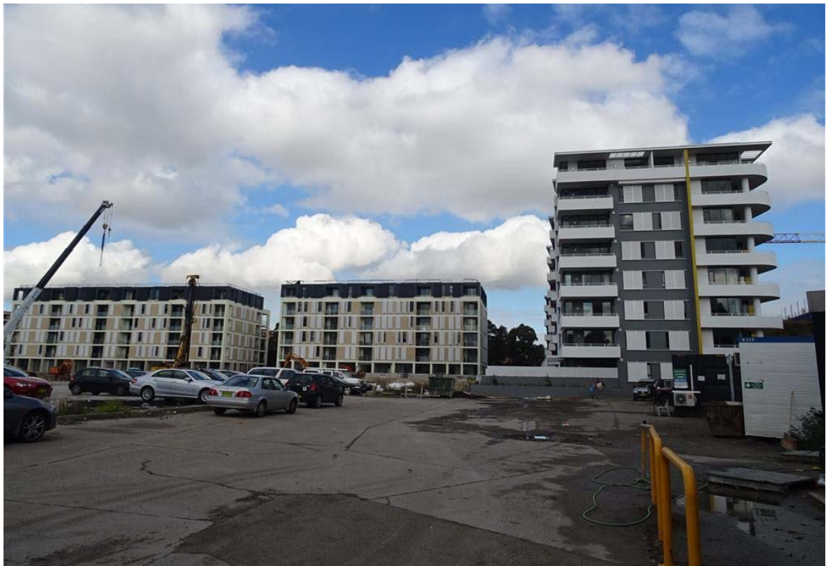
Figure 5: Looking south across the site showing Buildings H, G and D nearing completion.
